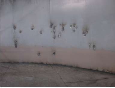
Corrosive spots on the walls of the Carnelian Woods #2 Tank
